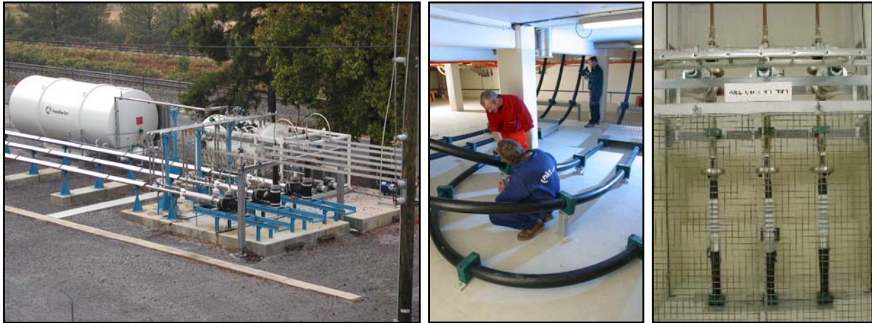
Figure 3 - Southwire (left) and nkt cables (middle & right) 30-m demo's
